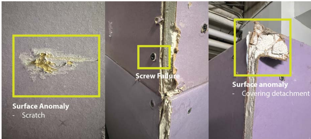
Figure 6.8: Three types of defects on the dry wall component. Image credit: Author.
